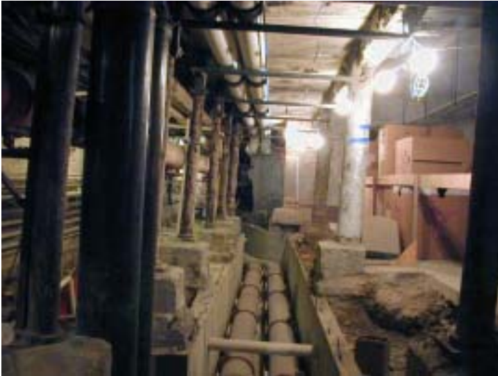
Figure 2- Distribution of chilled water was a difficult process, sometimes requiring pipe trenches
