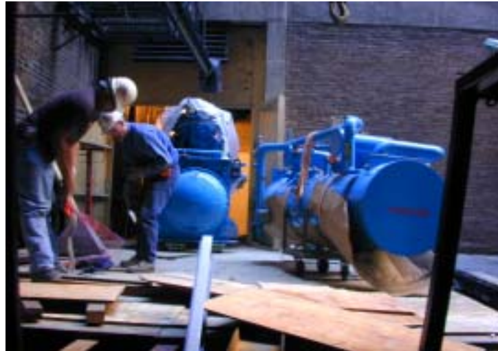
Figure 6 - Coordinating entry of all major equipment through a new masonry opening in the exterior of the building saved considerable construction costs. This new wall opening was
