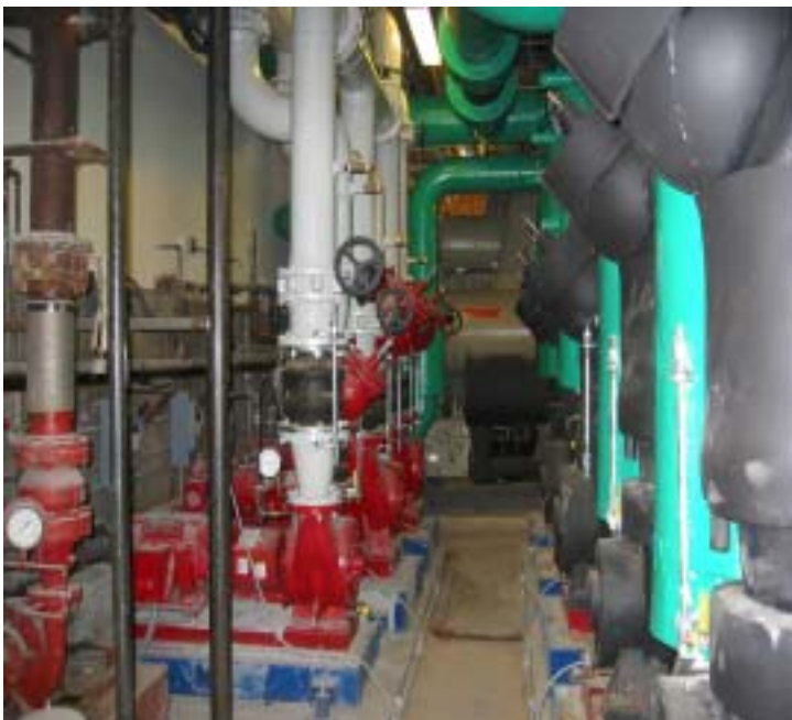
Figure 4 - New primary, secondary chilled water and condenser water pumping
