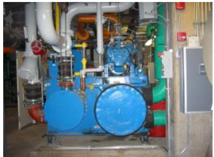
Figure 3 - A new gas engine drive chiller will provide significant operating savings and assisted in minimizing electrical requirements of the new cooling plant
