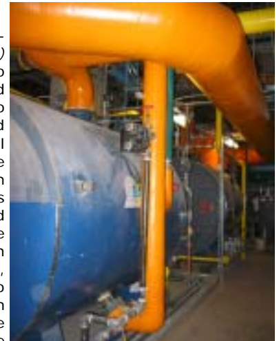
Figure 5 - New steam boilers more closely match partial load periods
