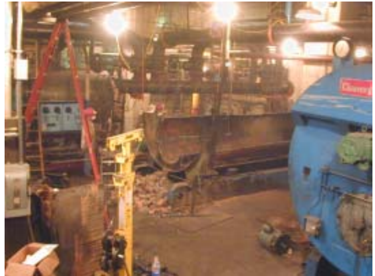
Figure 1 - The removal of a non-functional boiler provided space for the new cooling equipment
