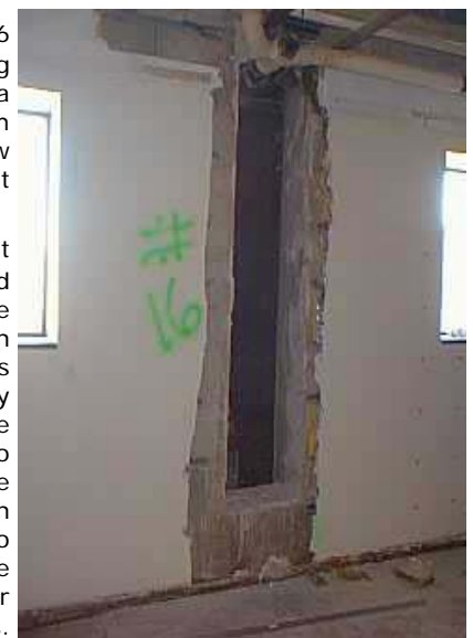
Figure 3-A 16" access to each exterior duct shaft was all that was available, limiting options on
