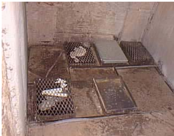
Figure 5-Inside the top of each exterior shaft, 4-6 lab exhaust ducts originally terminated in a plenum. Each plenum was served by one or two of the 56 original exhaust fans. A venturi style air valve was installed on each duct during the renovation, and connected to the new medium pressure lab exhaust system.
