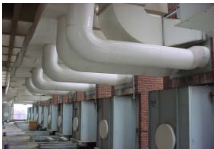
Figure 6- Photo after the 56 exhaust fans were demolished, with the building now served by new lab exhaust fans. Round white insulated ducts are return ducts serving certain duct risers within
