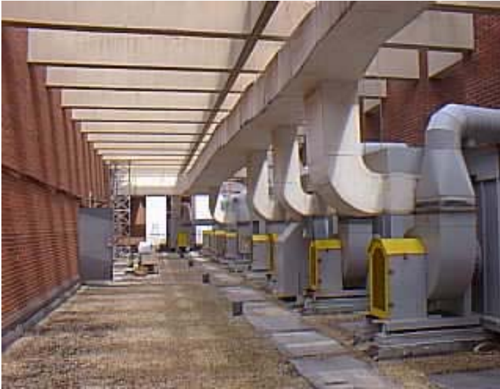
Figure 2 - Originally, the building was served by 56 lab exhaust fans. Each fan served four or five separate floors.
