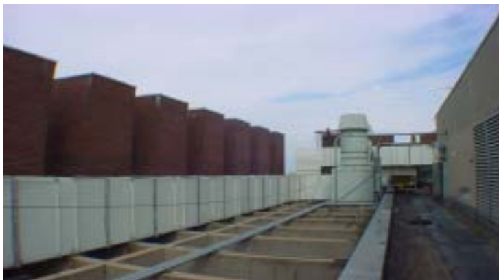
Figure 4-New lab exhaust fans were provided at each quadrant of the building and manifolded together by a
